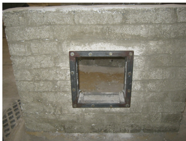
Figure (10) Details of the used rehabilitation technique using steel angle 3x30 mm around opening at both sides welded with steel angle inside opening corners.
