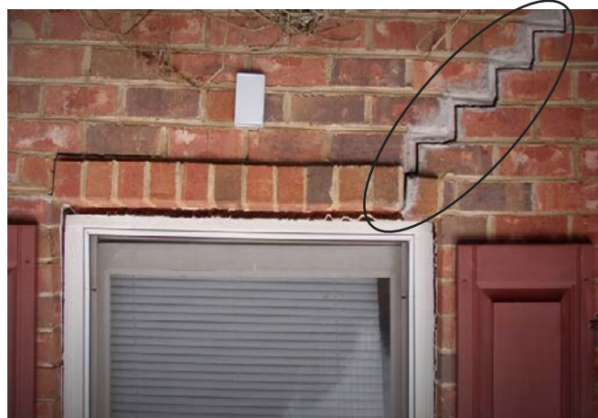
Figure (2) Diagonal cracks in brick wall.
