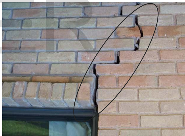
Figure (1) The cracks in brick wall with openings at filed
